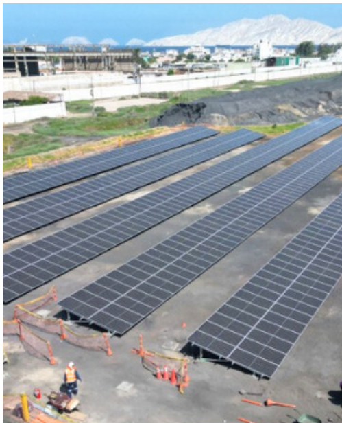
PV SIDER CHIMBOTE 500KWP
